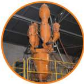
Autohoper Mixer in tape Plant
